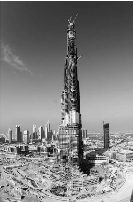
Figure 1.5 At this point in its construction, the super skyscraper Burj Dubai had already attained the title “world’s tallest building.” Courtesy of Samsung Engineering and Construction.
