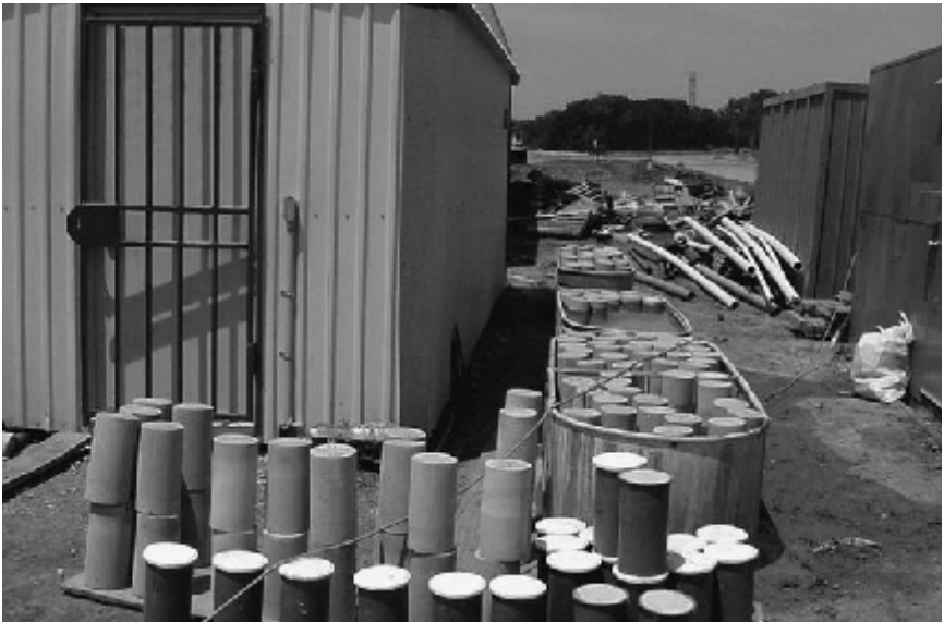
Figure 9.5 Improper storage of test cylinders at field laboratory.
