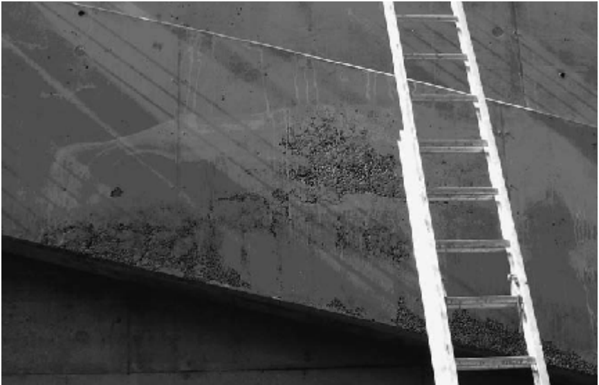
Figure 7.2 Honeycombs in monolithic spandrel beams placed integrally with deep, thin walls. This element was placed with a well-proportioned and adequately produced SCC mixture. These honeycombs developed because of excessive obstructions encountered during free fall into the formwork. The occurrence of honeycombing could have been reduced had the element been detailed in such a way that the top portion of the beam had been gradually chamfered (tapered) into the wall face. Courtesy of CTL Group.
