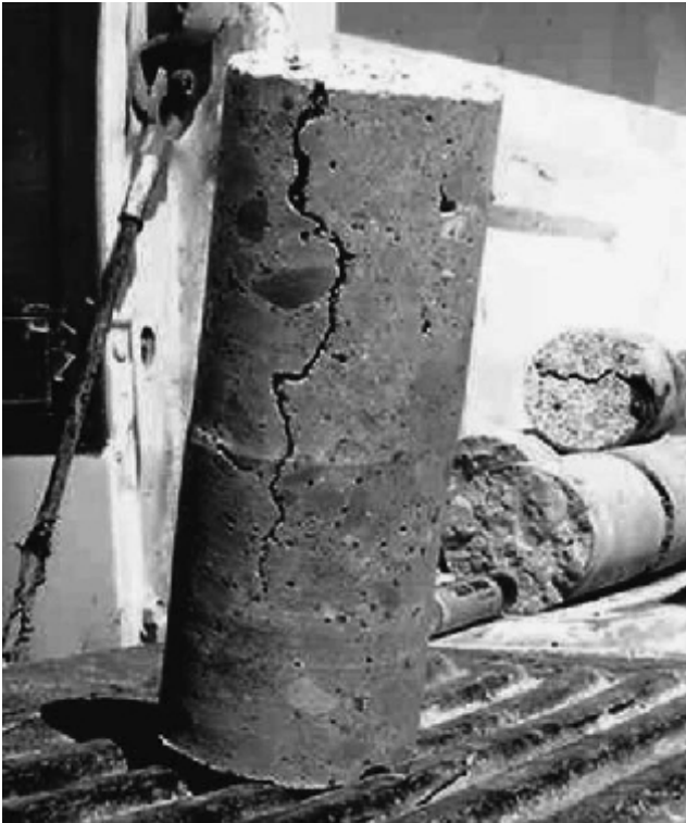
Figure 8.1 Severe plastic shrinkage cracking caused by ineffective interim curing. Cracks of this nature start out relatively shallow, but subsequently are capable of behaving as contraction joints, causing the cracks to propagate deeper into the section. Courtesy of CTL Group.
