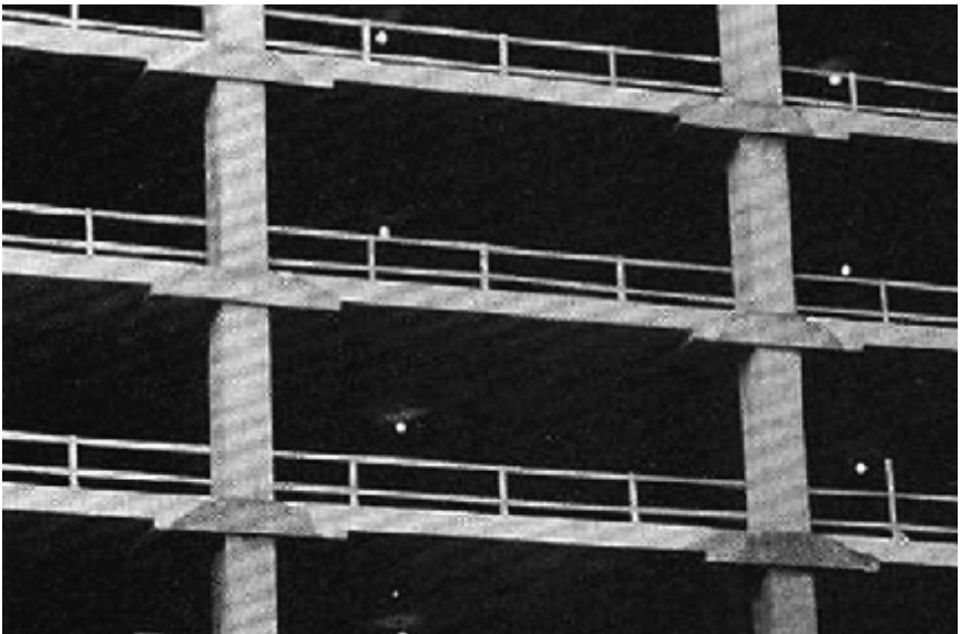
Figure 10.11 Color contrast of darker column concrete (containing silica fume), with slab concrete. Courtesy of American Concrete Institute.
